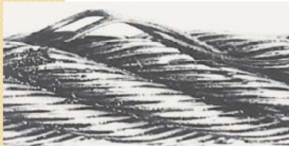
Wire fractures at the strand, or core interface, as distinct from ‘crown’ features
